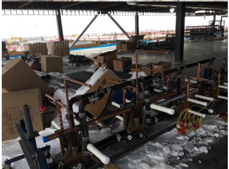
Photo 3: Main floor: Plumbing core for restrooms is on-site. Notice slab is poured.
