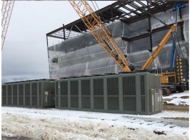
Photo 2: Material on-site: Roof-top mechanical equipment on-site.
