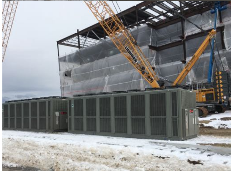
Photo 2: Material on-site: Roof-top mechanical equipment on-site.
